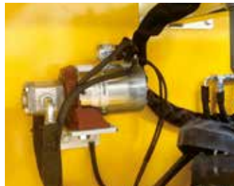
Emergency electric pump
